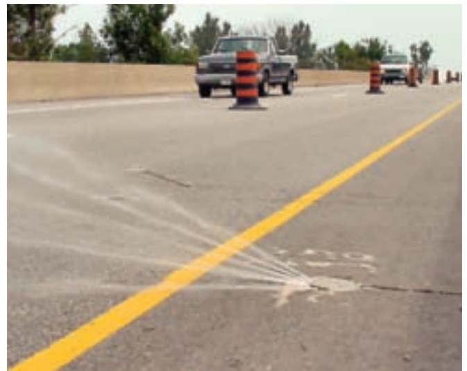
Pavement-mounted anti-icing sprayers can be remote-operated if an RWIS indicates an icing event is imminent.
