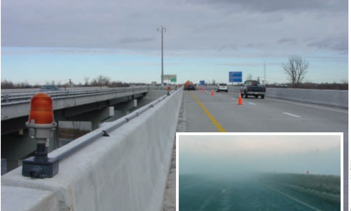
Barrier-mounted fog warning lights (above) are useful in guiding traffic through fog-shrouded highways (inset).
