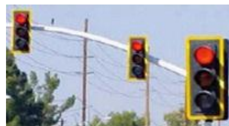
Figure 13. 3 in. retroreflective borders on signal backplates (FHWA 2011)
