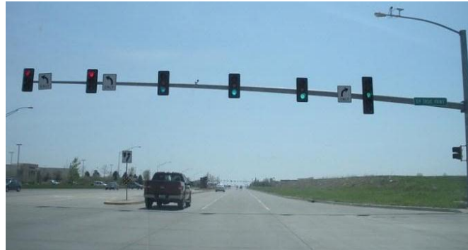
Figure 4. Example of one signal head per lane at Jordan Creek Parkway and EP True Parkway in Des Moines, Iowa
